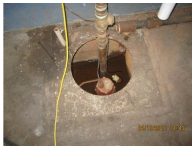
Boiler Room Sump Pump
