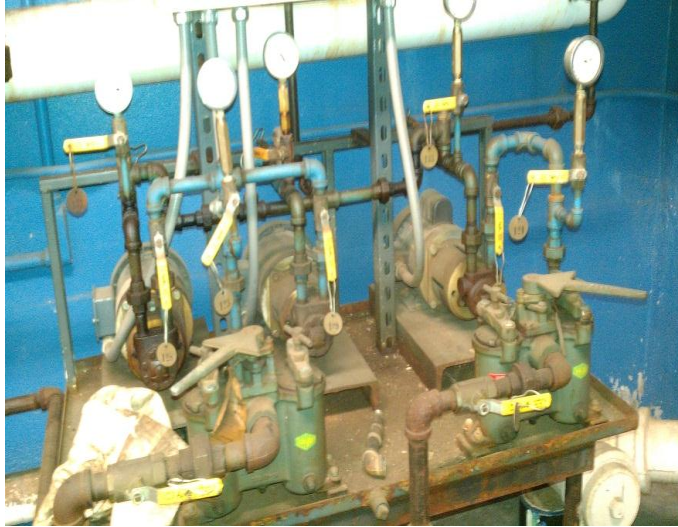
Fuel Oil Pumps & Piping
