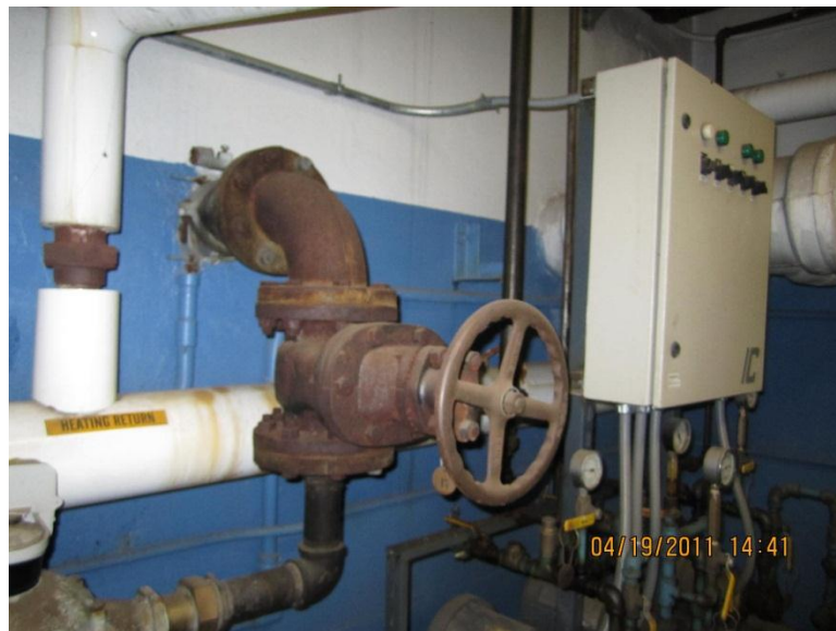
Water Service Entry
