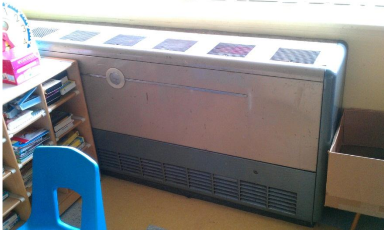
Very Old Classroom unit Ventilator
