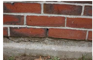
Image 3: Cracks in foundation wall
