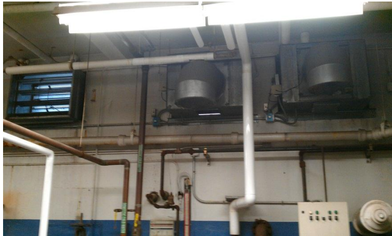
Boiler Room Ventilation/Combustion Air Intake & Exhaust
