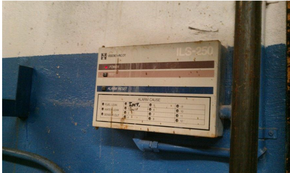
Old Veder-Root Tank Monitoring System
