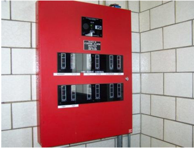
Main Fire Alarm Control Panel
