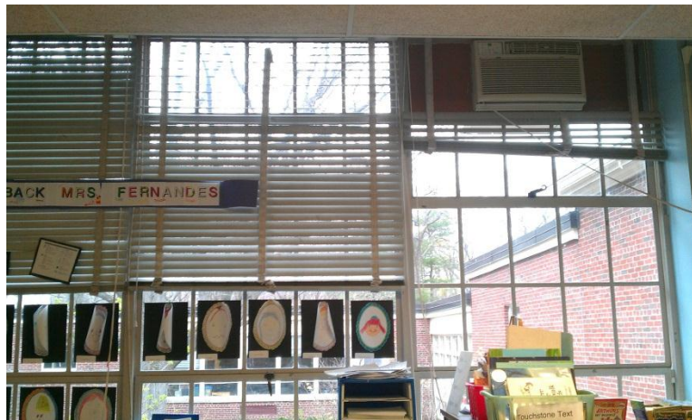
Window Air Conditioner Installed In Operable Window Space
