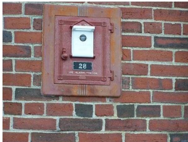
Fire Alarm Masterbox
