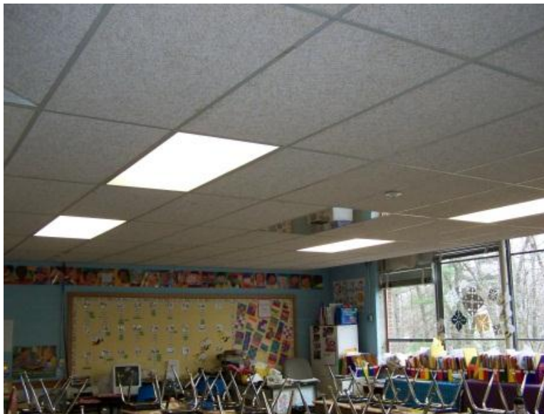
Classroom and Office fixture
