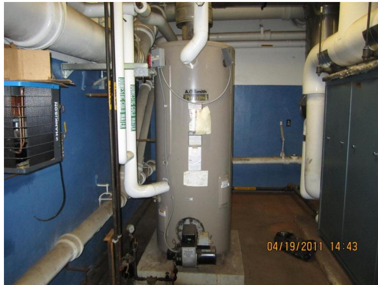
Domestic Water Heater
