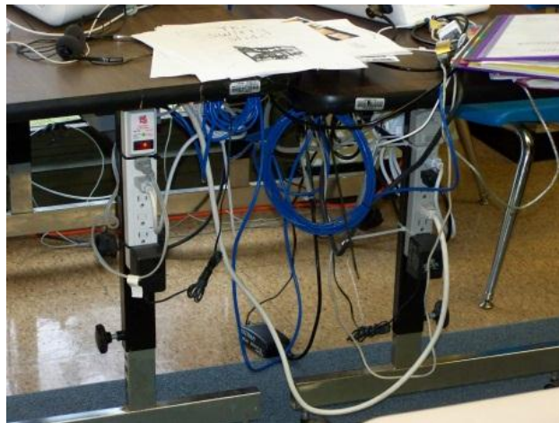
Photo 9: Typical Technology Receptacle
