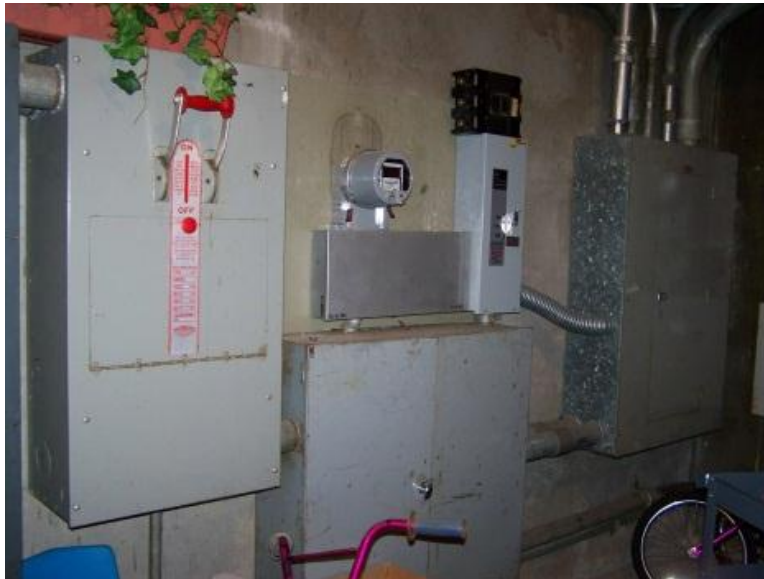
Main Service Equipment
