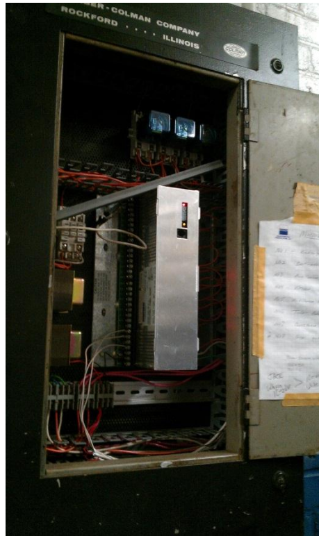
Barber-Colman Network 8000 DDC control System
