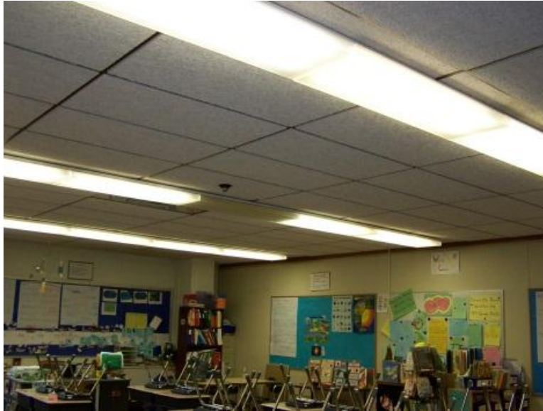
Classroom Fluorescent Fixtures
